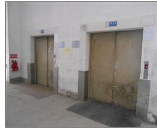
Photo of non-conformity No warning sign near the cargo lift.JPG
