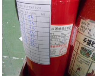
Photo of fire safety equipment Inspection tag for fire extinguisher.JPG
