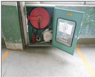
Photo of fire safety equipment Fire hydrant.JPG
