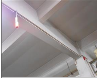
Photo of fire safety equipment Fire alarm.JPG
