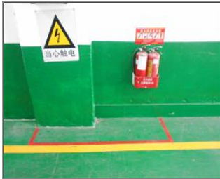
Photo of fire safety equipment Fire extinguishers.JPG
