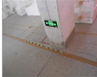
Photo of fire safety equipment Lighting evacuation sign along the evacuation passage.JPG
